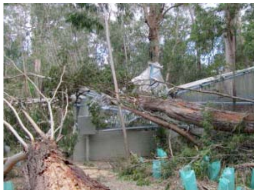
Damaged orchid house
